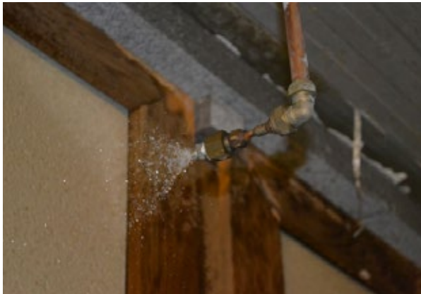
Fig 4 Water being sprayed onto the face of a ModCell® Traditional Panel
